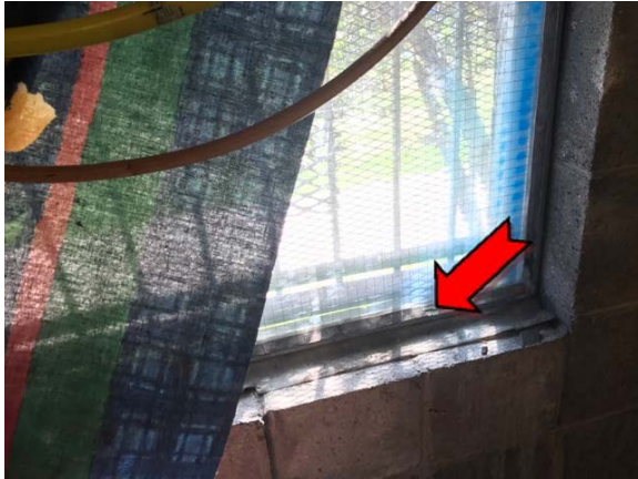
Photo Interior, throughout, window frames – 1. asbestos-containing caulking material.
